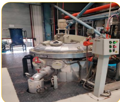
Autoclave for vacuum drying & oil impregnation.
